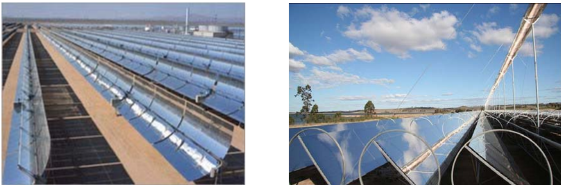
Figure 5. Parabolic trough (left) and linear Fresnel (right) collector systems (photos from http://en.wikipedia.org/wiki/Solar_thermal_energy ).
